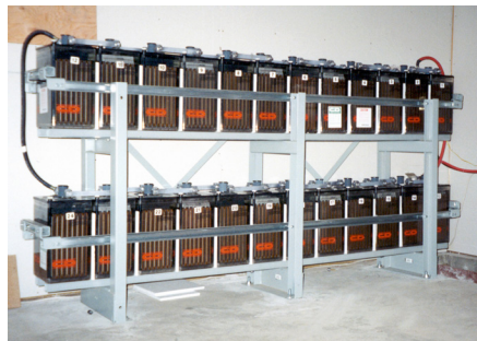
Battery bank for an off-grid home solar power system.
