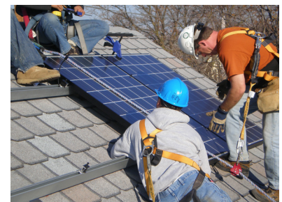
Crystalline solar modules mounted on aluminum racks, with airspace to keep them cooler.
