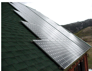
Monocrystalline solar panels.
